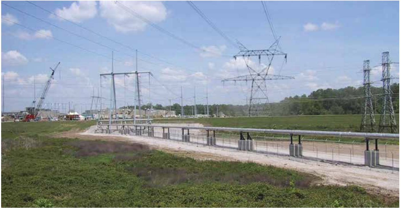
Baxter Wilson Power Plant, Mississippi, USA 550kV, 3000A Grid Connection Across Transmission Lines
