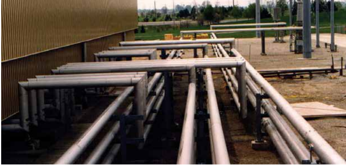
Claireville Transmission Station, Ontario, Canada 250kV Bus Line Exits
