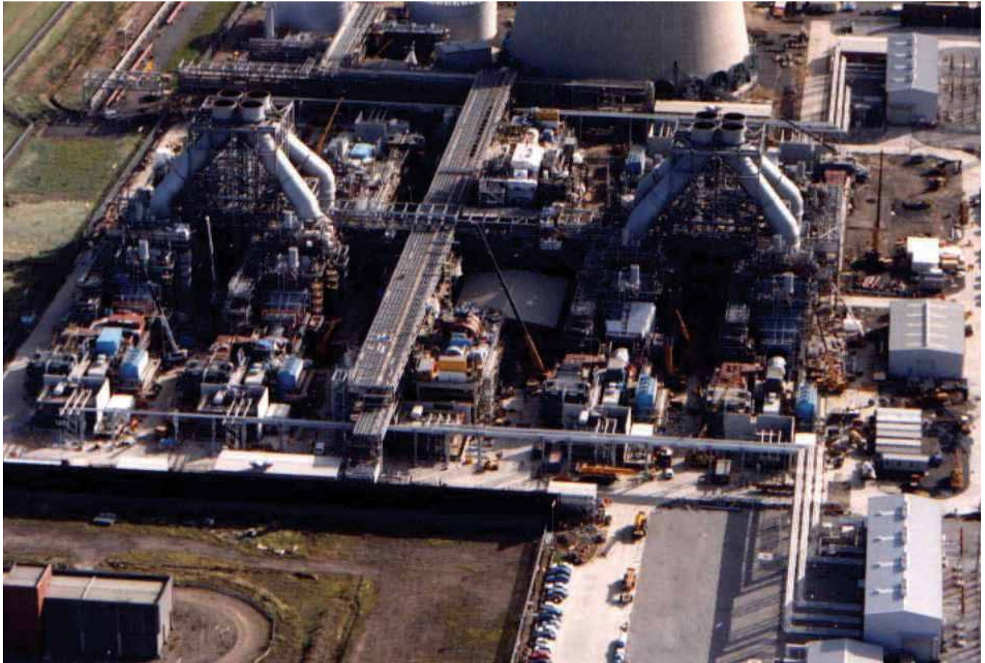
Teesside Combined Cycle Power Plant, England 275kV GIL Connections Between Generator Step-up Transformers and GIS Building
