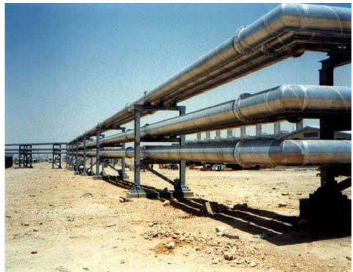
Power Plant 8, Saudi Arabia 380kV, 1200A GIL System Installed Above Ground
