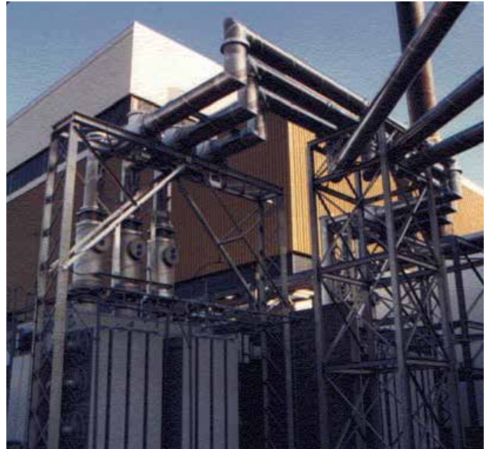
Seabrook Nuclear Power Plant, New Hampshire, USA 345kV, 3000A Combined trench and above ground Installation
