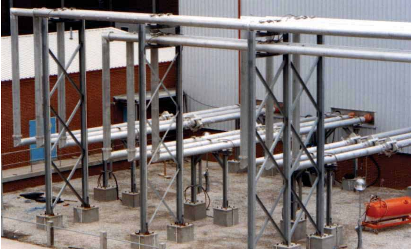
Teesside Combined Cycle Power Plant, England 275kV GIL Elevated Connection Circuits
