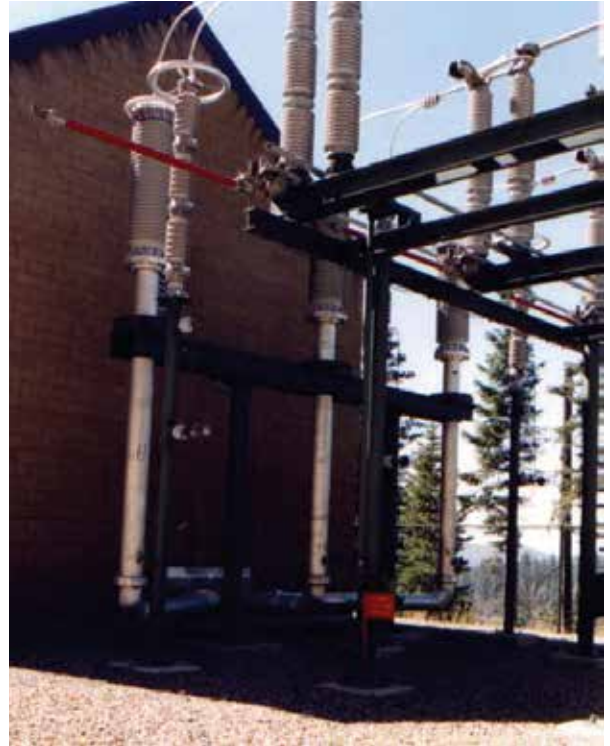
Balsam Meadows Pumped Storage Plant, California, USA 230kV GIL Exit From Top of Shaft Enclosure Building to Overhead Line Bushings
