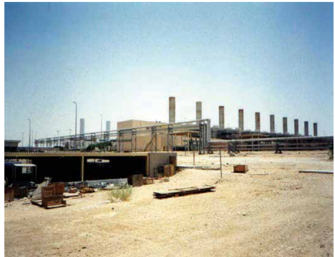
Power Plant 8, Saudi Arabia 380kV, 1200A GIL System Connecting to Transformers
