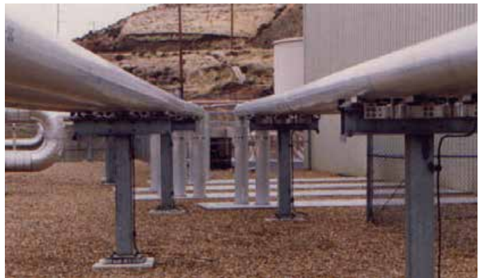
Midway Sunset Cogeneration Plant, California, USA 242kV, 2000A Combined Trench and Above Ground Installation
