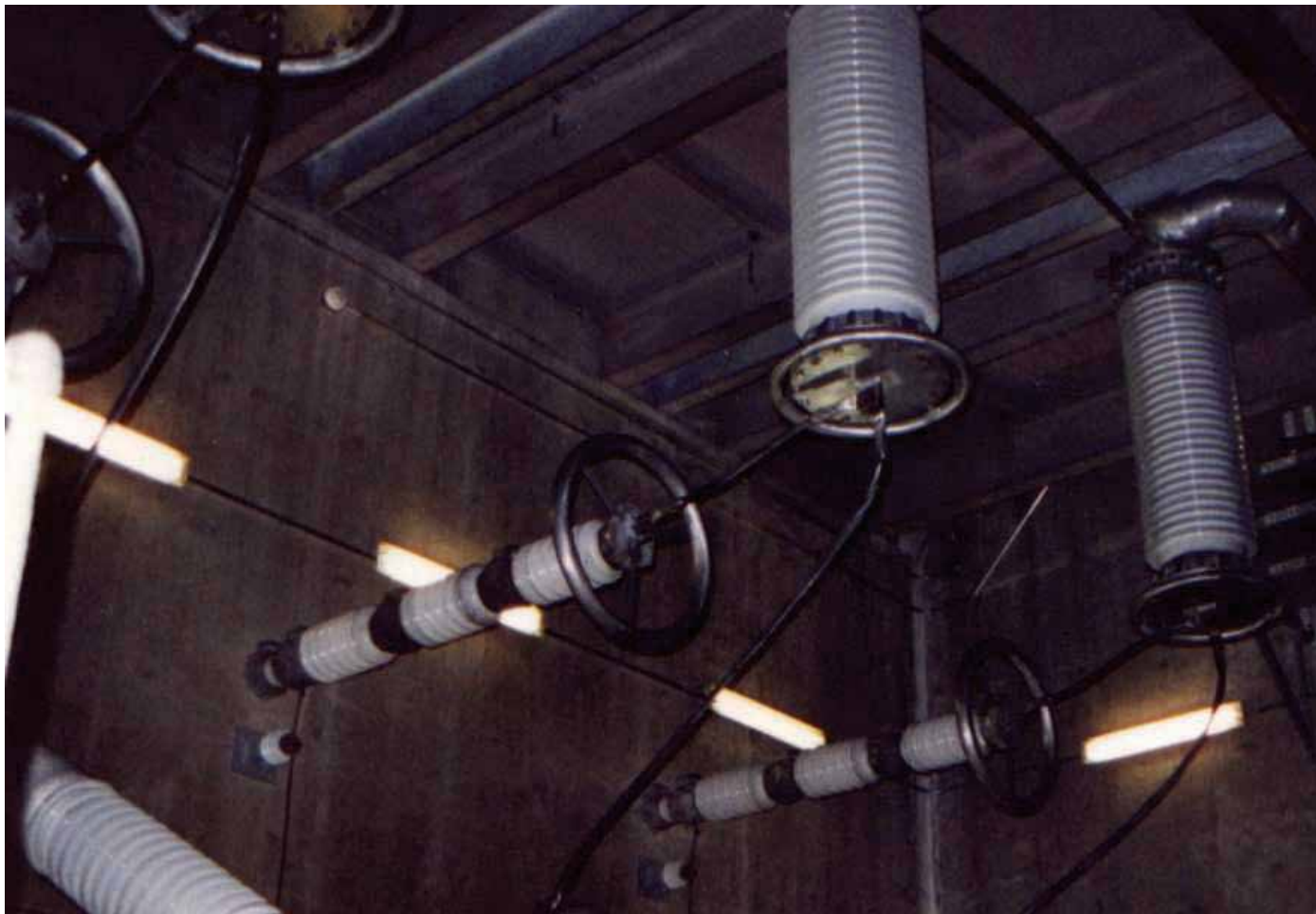
Balsam Meadows Pumped Storage Plant, California, USA 230kV GIL Bushings Installed in Transformer Room
