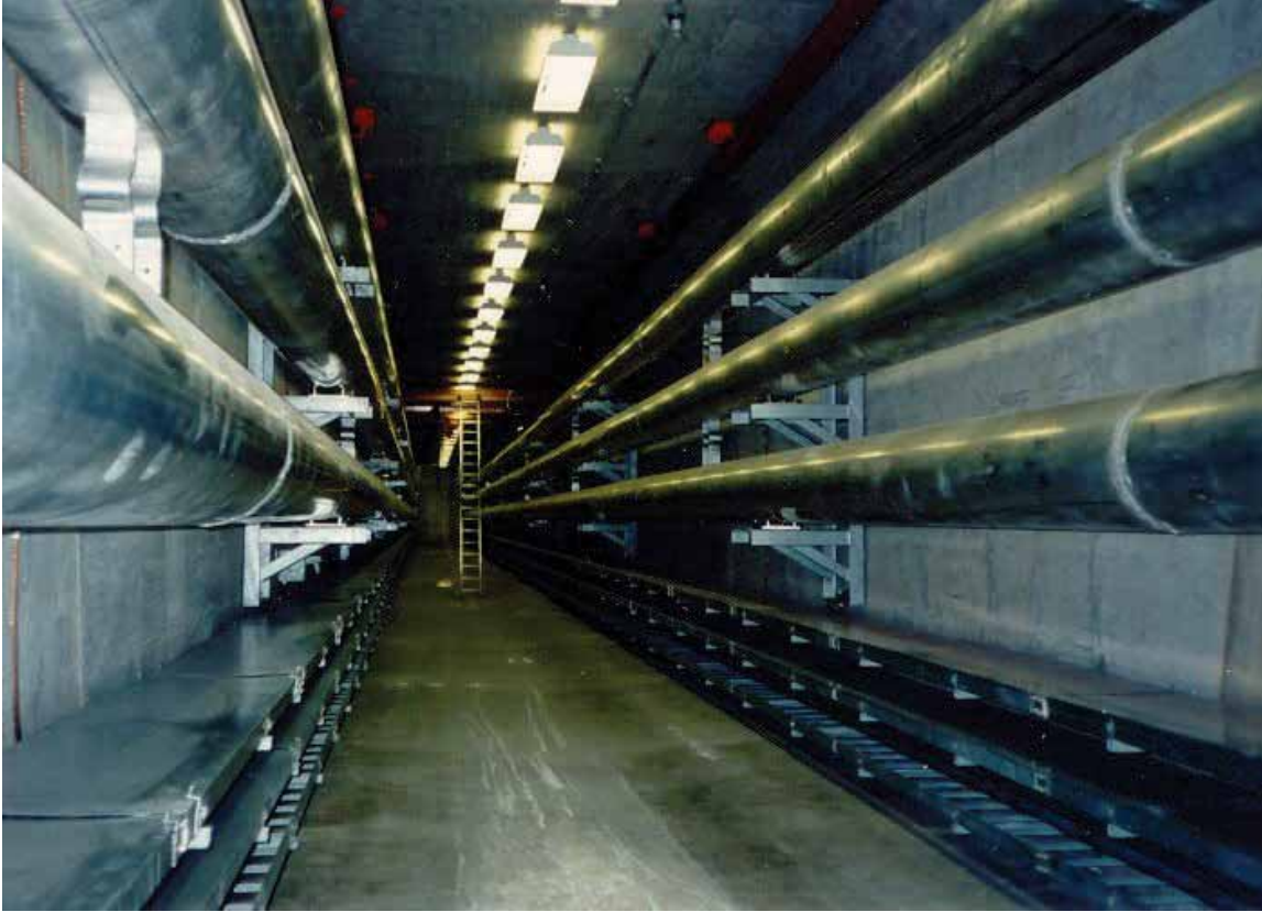
Revelstoke Hydroelectric Project, British Columbia, Canada 550kV, 4000A GIL Installed in Inclined Tunnel
