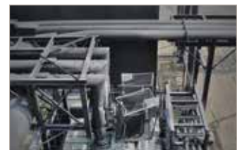
The impact of high temperatures at the transformer connections.
