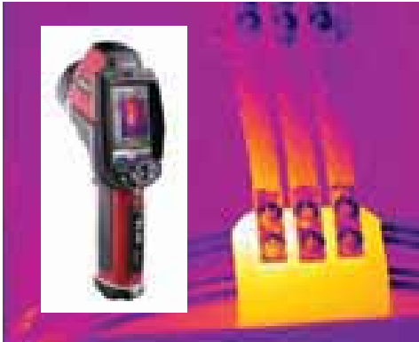
Hot spots shown in thermal analysis can pinpoint loose or broken connections before they become an issue.
