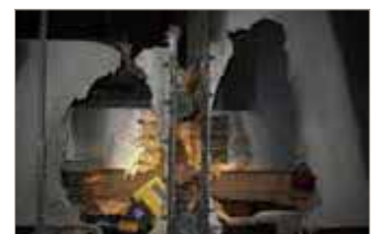
The impact of loose connections at the flex terminations.
