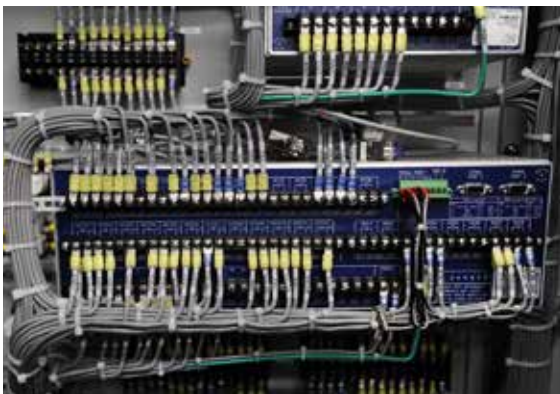
The installation of our customized wiring sets the industry standard for quality and efficiency
