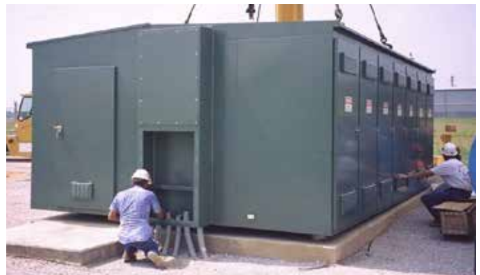
Our Field Services Team provides unmatched service and experience
