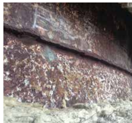
Full circumferential skirt cracks
